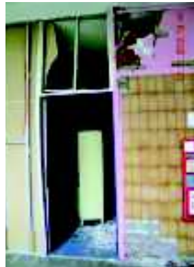
Figure 15. Damage at Felix Bulnes Hospital, outside of Santiago. As of July 2010, the hospital was still partially closed due to unrepaired damages.
